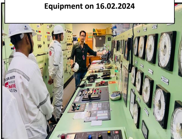
Engineer Control Room familiarization on 16.02.2024
