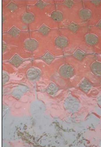
Rainwater recharging through open pavers
